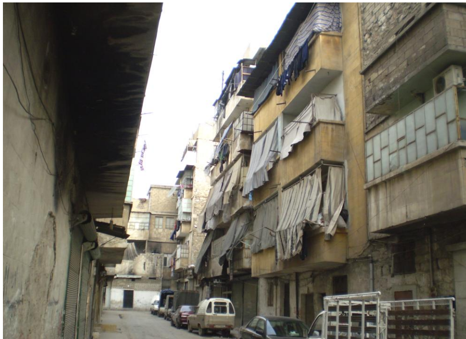
Crudely screened balconies on an apartment building in Damascus, Syria. Obviously, the people embraced some utilitarian ends at the expense of the aesthetic ones.
