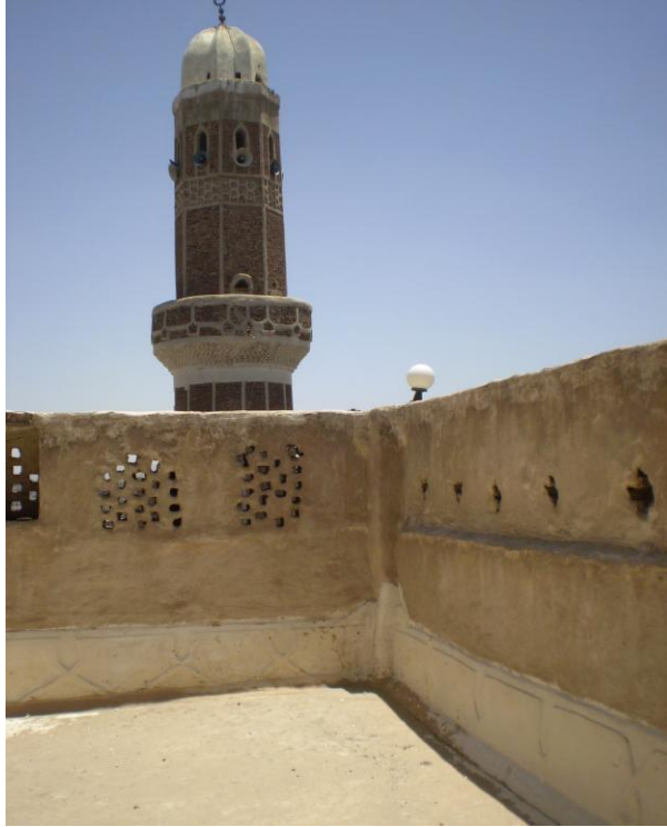
A well protected open roof by a parapet in a house in San'a, Yemen.
