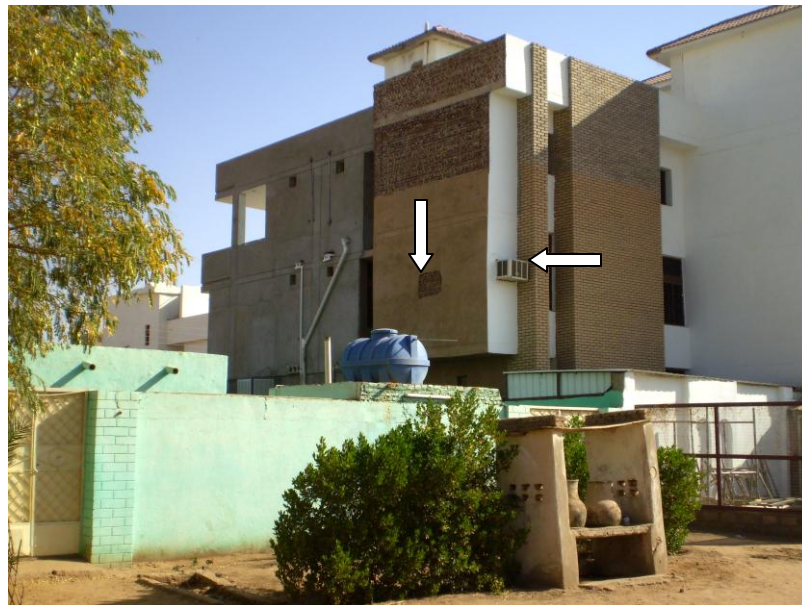
After a man in Khartoum, Sudan, had complained to his neighbor that an air conditioner fixed on the latter's façade that faces the former's courtyard house causes him and his household a problem with regard to noise, potential pollution and even privacy, the air conditioner was moved away to the side of the house that faces a street. The opening which at first was meant for the air conditioner was then duly bricked up -- as shown in the picture.
